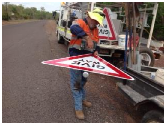
Signage replaced due to damage and vandalism
