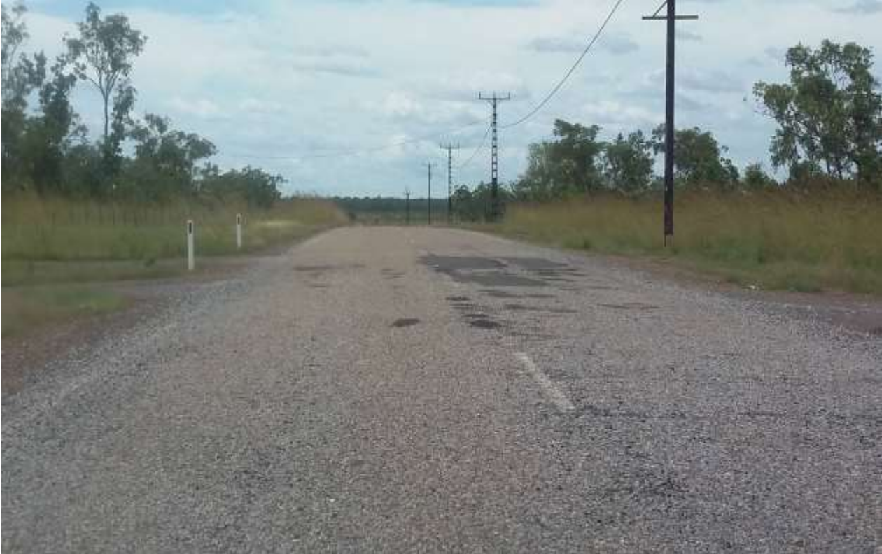
Figure 3 - Sealed road requiring renewal
